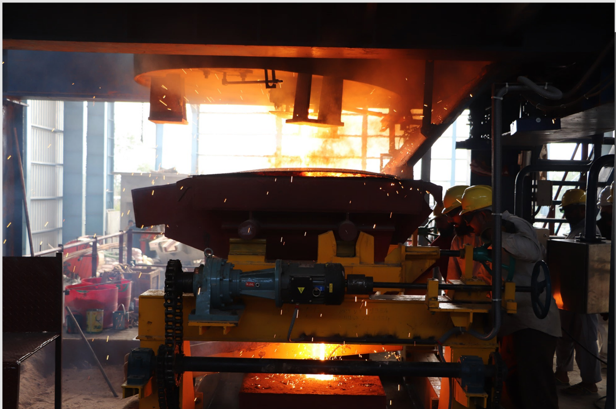
From ladle to tundish & from tundish to CCM, a mesmerizing view of molten metal at 1600 °C passing into the CCM on the first day of commercial production.
